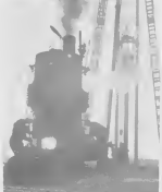
MORE THAN 2700 timber piles were driven in the soft earth to form foundations for heavy refinery structures. MAS DI 2700 pilon a worde manda den e suelo moli pa forma fundeshi di e structuranan piad di refinaria.
